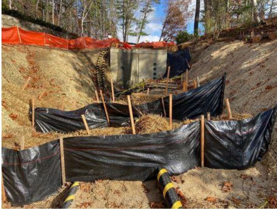
Photo 7. Cable trench, facing manhole, view northeast, Newington, NH.
