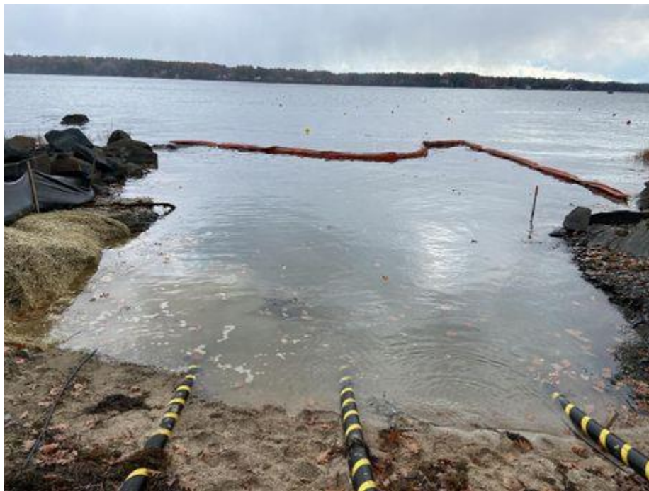
Photo 2. Turbidity barrier installed at edge of cable install, view east, Durham, NH.
