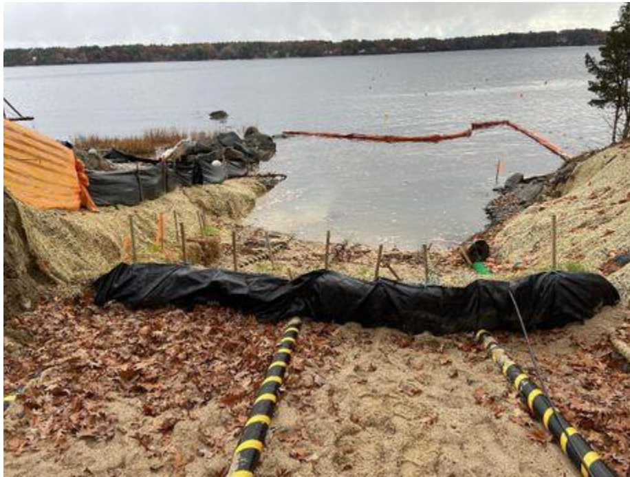
Photo 1. Cable trench, view of silt fence/straw bail barrier at edge of underwater cable crossing, facing east, Durham NH.
